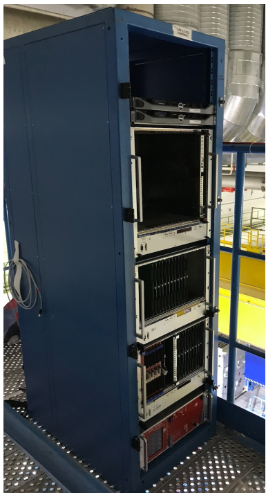
DAQ rack: without cabling
