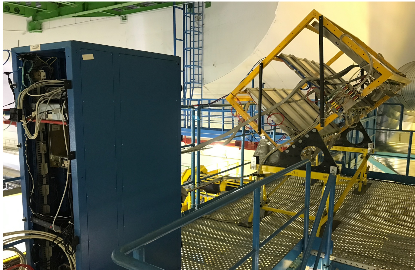
proANUBIS + DAQ rack installed in their positions within the ATLAS experimental Cavern (Level 12 of UX15)
