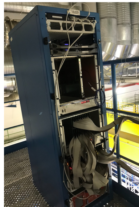
DAQ rack: fully cabled-up
